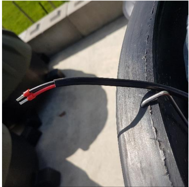
Connections for High Level Alarm
