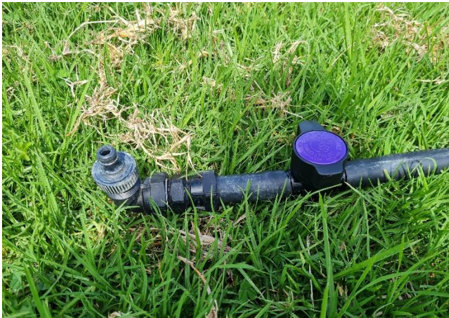
End flush tap and hose connection.
